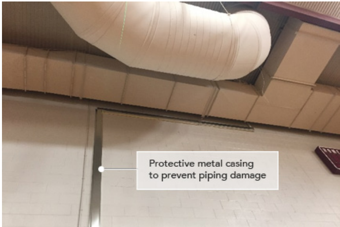
DRAIN PIPING WITH PROTECTIVE CASING
