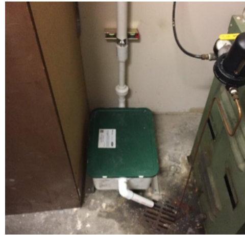
CONDENSATE NEUTRALIZER INSTALLED
