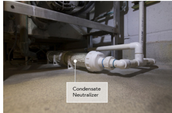
CONDENSATE NEUTRALIZER INSTALLED
