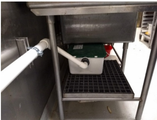
CONDENSATE NEUTRALIZER TANK
