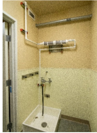
CONDENSATE NEUTRALIZER INSTALLED
