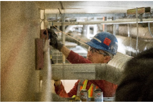
CONDENSATE DRAIN PIPING
