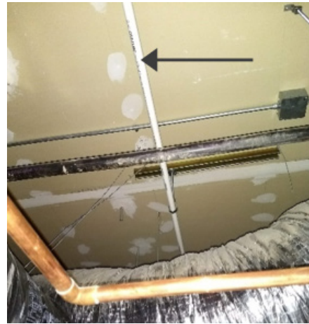
CONDENSATE DRAIN PIPING
