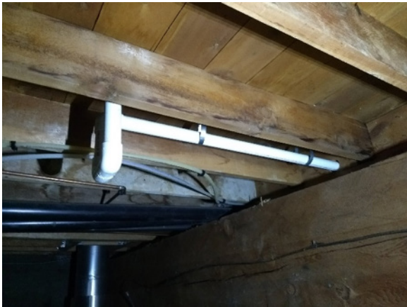
DRAIN PENETRATION & P-TRAP BELOW UNIT
