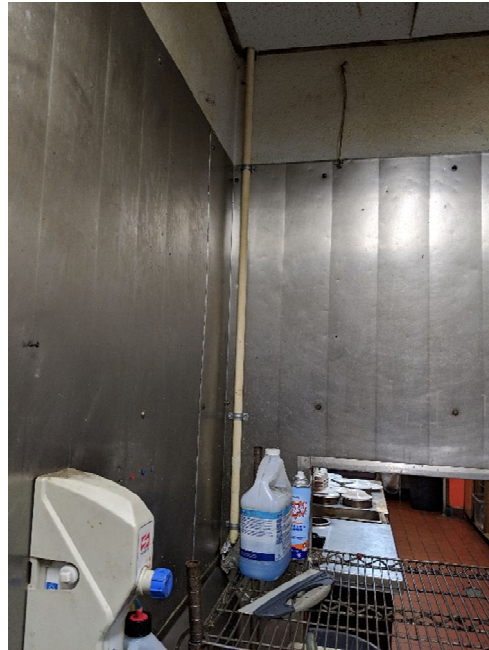
CONDENSATE LINE TERMINATING IN KITCHEN SINK
