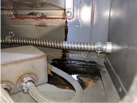
FIGURE 18 – SITE A FLUE BOX LEAK
