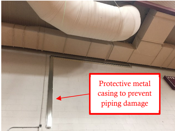
DRAIN PIPING WITH PROTECTIVE CASING
