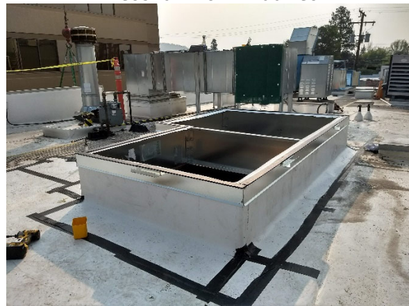
NEW CUSTOM-BUILT ROOF CURB
