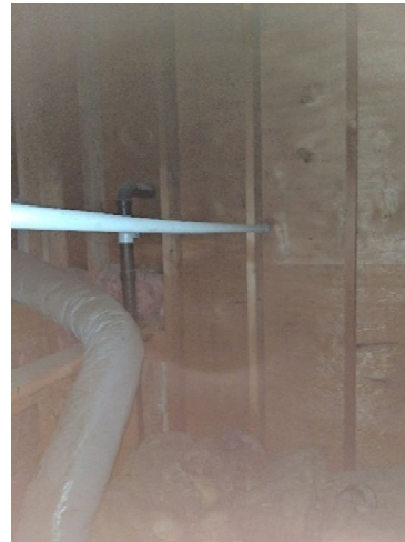
UNNEUTRALIZED CONDENSATE PENETRATION IN TOILET VENT PIPE
