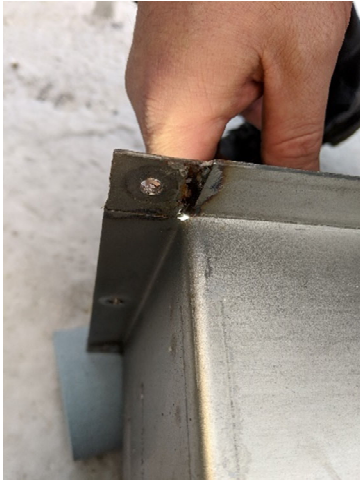
FIGURE 20 – SITE A FLUE BOX WELDING GAP & ORIGIN OF LEAK
