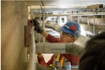
CONDENSATE DRAIN PIPING
