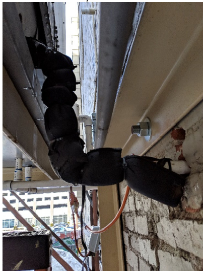
HEAT TRACE AROUND CONDENSATE LINE BETWEEN UNIT/BUILDING
