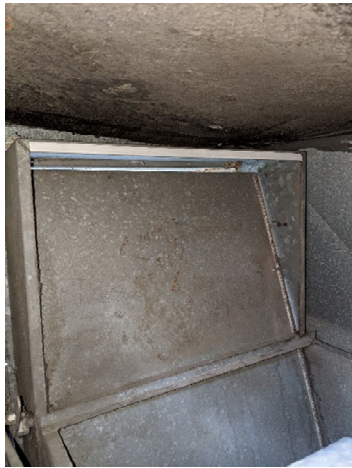
OUTSIDE AIR DAMPER CLOSED
