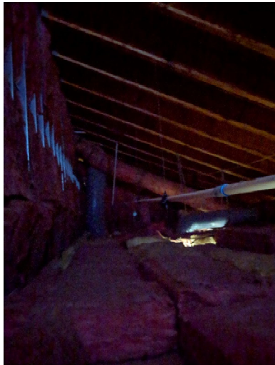
CONDENSATE DRAIN RUN IN ATTIC
