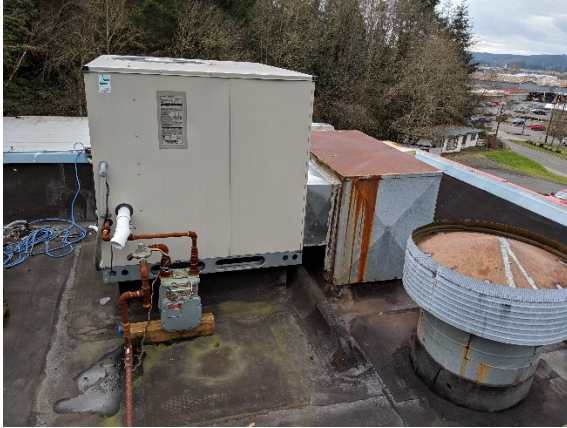
SITE B CONDENSING UNIT
