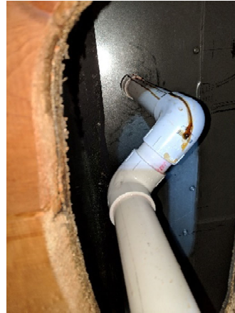
FIGURE 19 – SITE A LEAK INTO ATTIC SPACE
