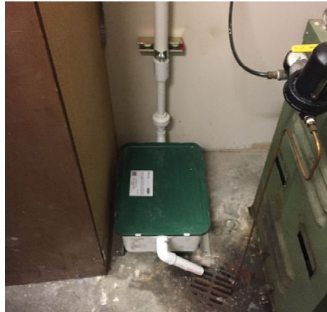
CONDENSATE NEUTRALIZER INSTALLED
