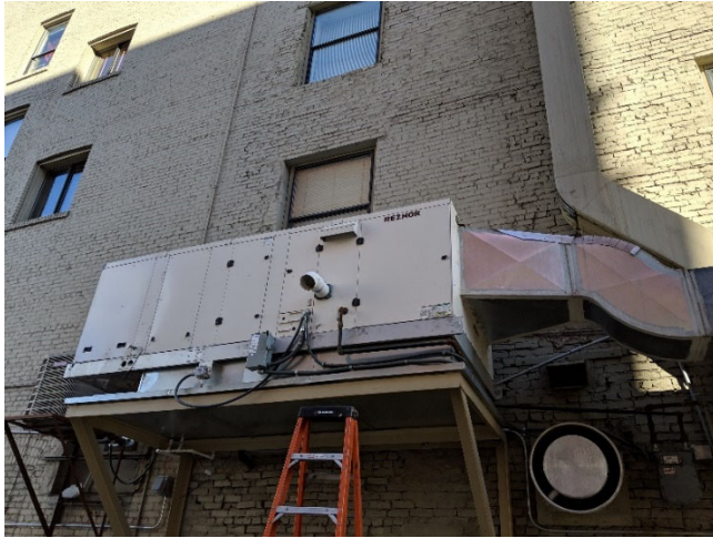
SITE D UNIT INSTALLED ON PLATFORM
